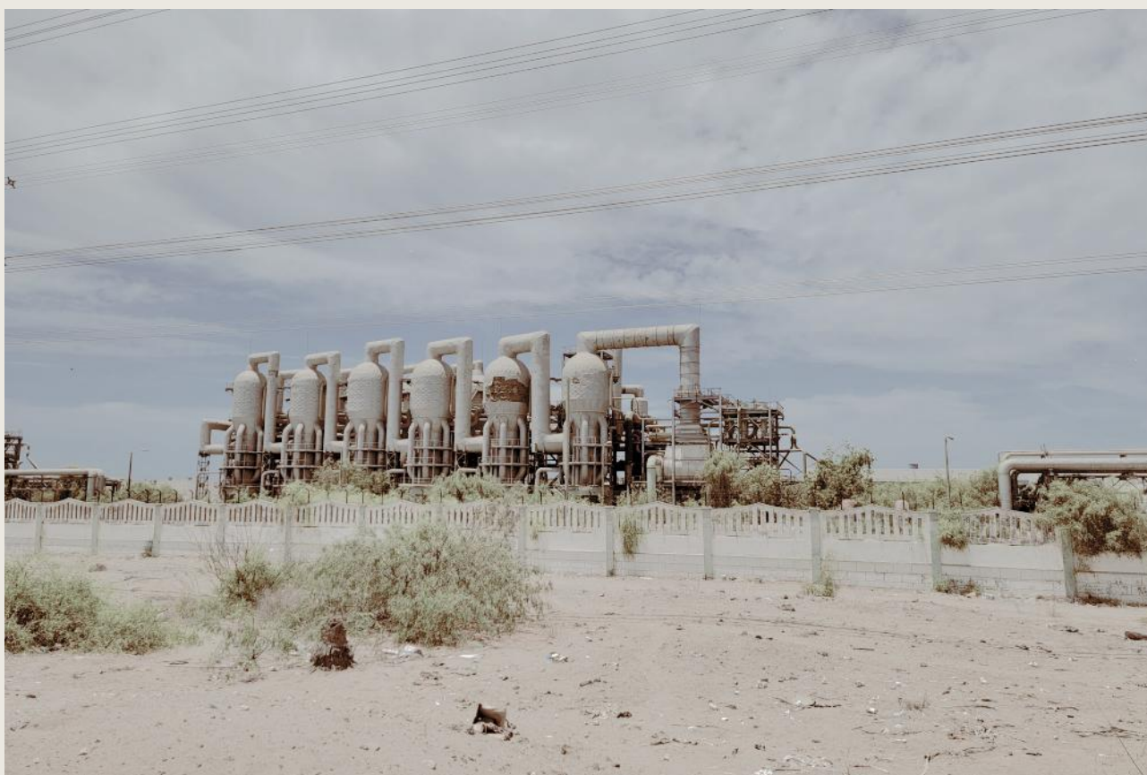
A POWER STATION IN ADEN, YEMEN, WHERE A SCORCHING HEAT WAVE AND PROLONGED ELECTRICITY OUTAGES HAVE PLUNGED RESIDENTS OF THE SOUTHERN PORT CITY INTO A STRUGGLE FOR SURVIVAL. © PICTURE ALLIANCE / XINHUA NEWS AGENCY | MURAD ABDO. 2023.
